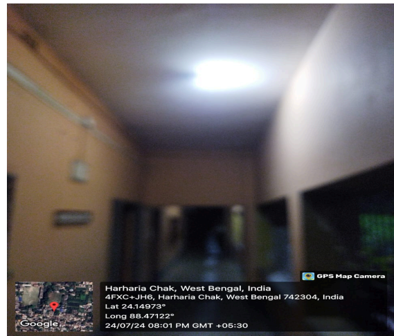
LED light in corridor
