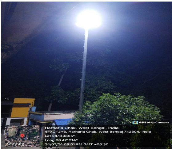
College uses high mast low voltage light.
